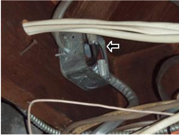
5.3 Picture 1 missing cover
