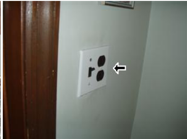
5.5 Picture 2 rec. GFCI
