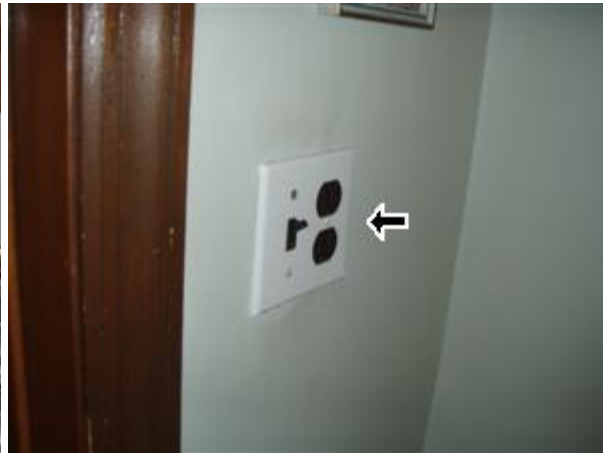
5.5 Picture 2 rec. GFCI
